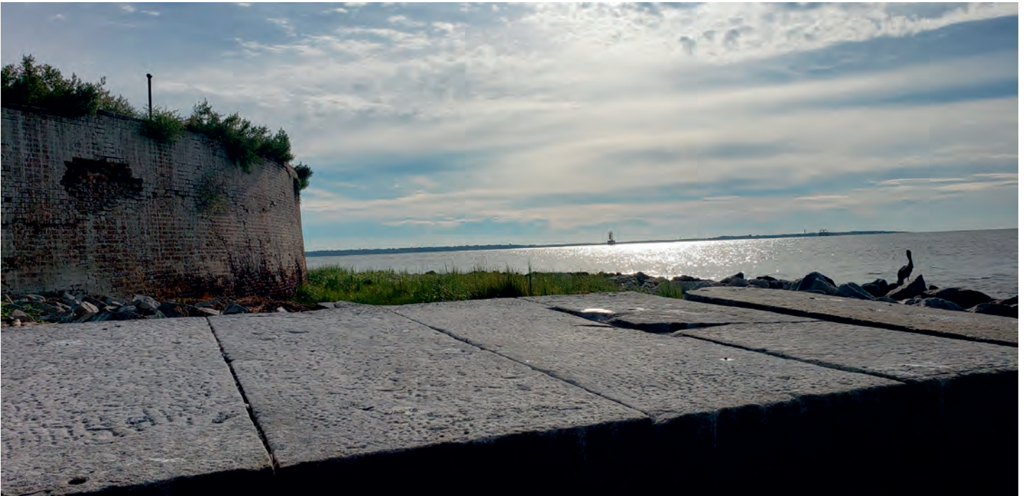
Figure 3: View from the original wharf showing the condition of the War of 1812-period walls. (Photo by John Fisher)
